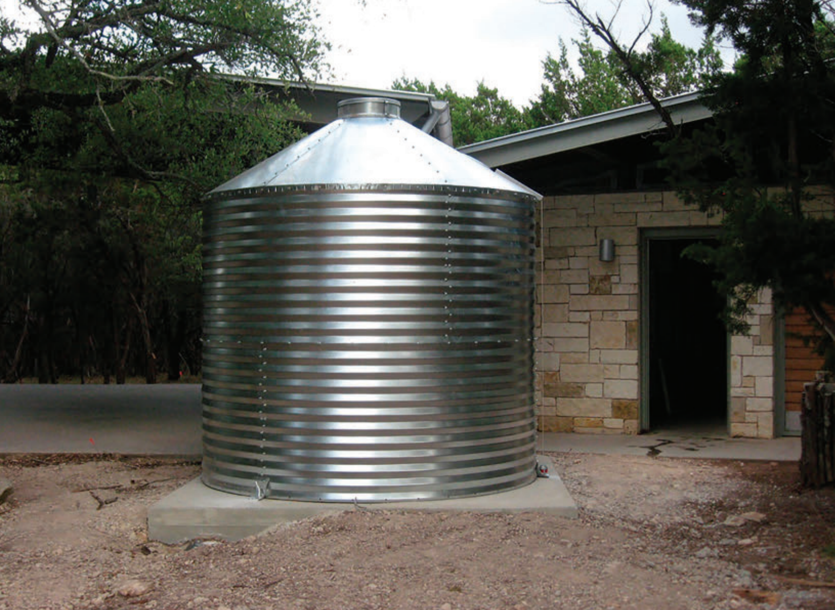
Blue Hole rainwater harvesting tank
