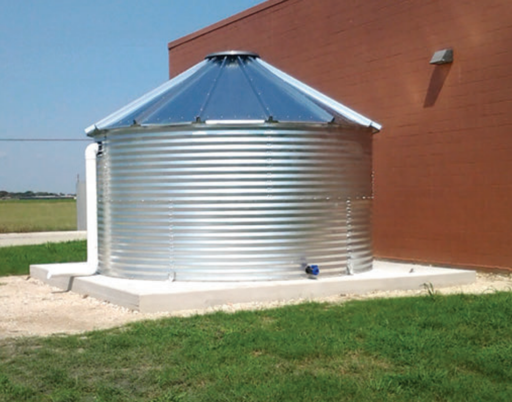
Caldwell County Justice Center rainwater harvesting cistern capable of catching and storing 10,000 gallons of rainwater
