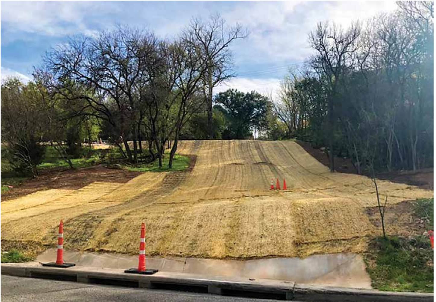
Matthews Street after installation of Hogtrap BMP. Photo courtesy of Aspen Navarro.
