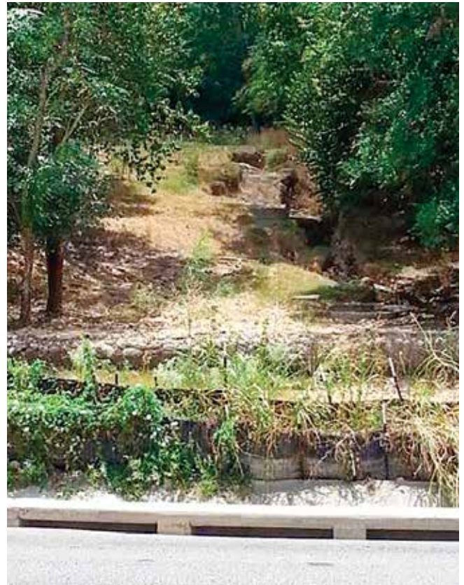
Matthews Street prior to installation of Hogtrap Best Management Practice (BMP). Photo courtesy of Aspen Navarro.
